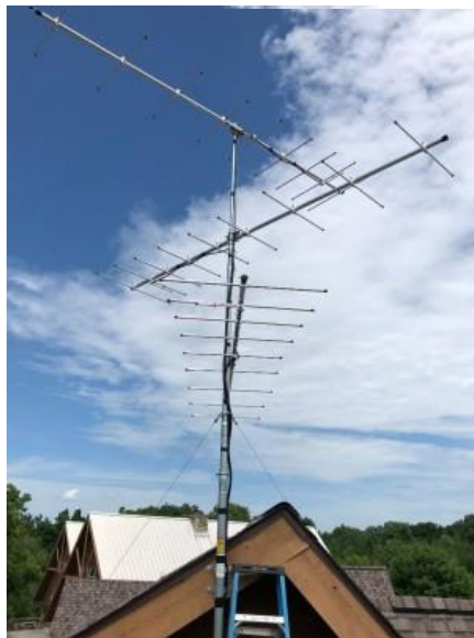
Example of Motus antenna mounted next to a building.
